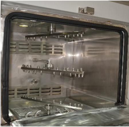
Big cleaning room
